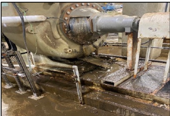
Sludge around the base of the packed pump.
